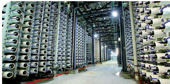
Figure 1: The scale of modern RO plants, such as the Ashkelon plant, Israel is remarkable (photo courtesy of Veolia Photo Library, R Mas)
